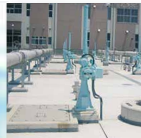
Water purification plant
